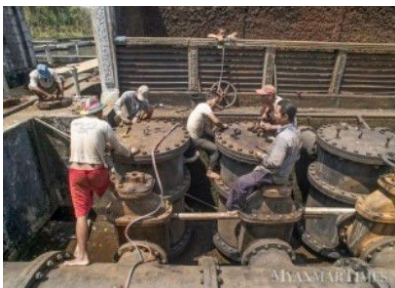
On track to meet Yangon's growing water needs
